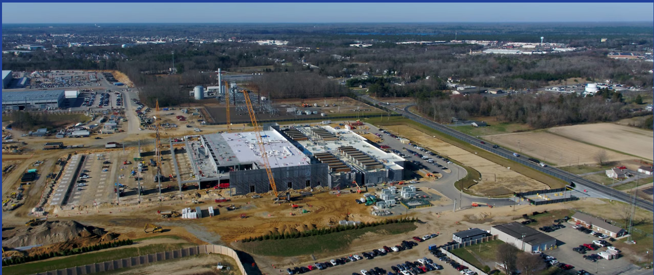
Aerial view of Vineland DataOne site during construction, showing site development and infrastructure installation
