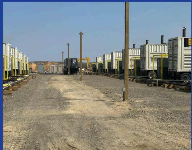
Temporary generator fleet supporting 100 MW phased energization
