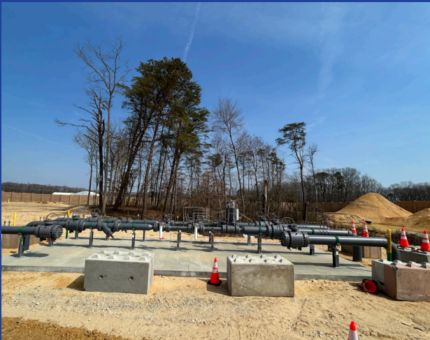
12" steel natural gas pipeline station supporting permanent infrastructure
